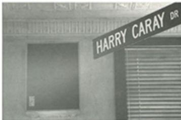
Modular Sound System engineers dealt with the problem of an inappropriate ceiling and limited wall space by custom designing shallow Bag End TA12 cabinets to house SE1280 speakers and E350 horns. The cabinets are mounted between the windows, and are finished to match the rest of the décor in the room.
